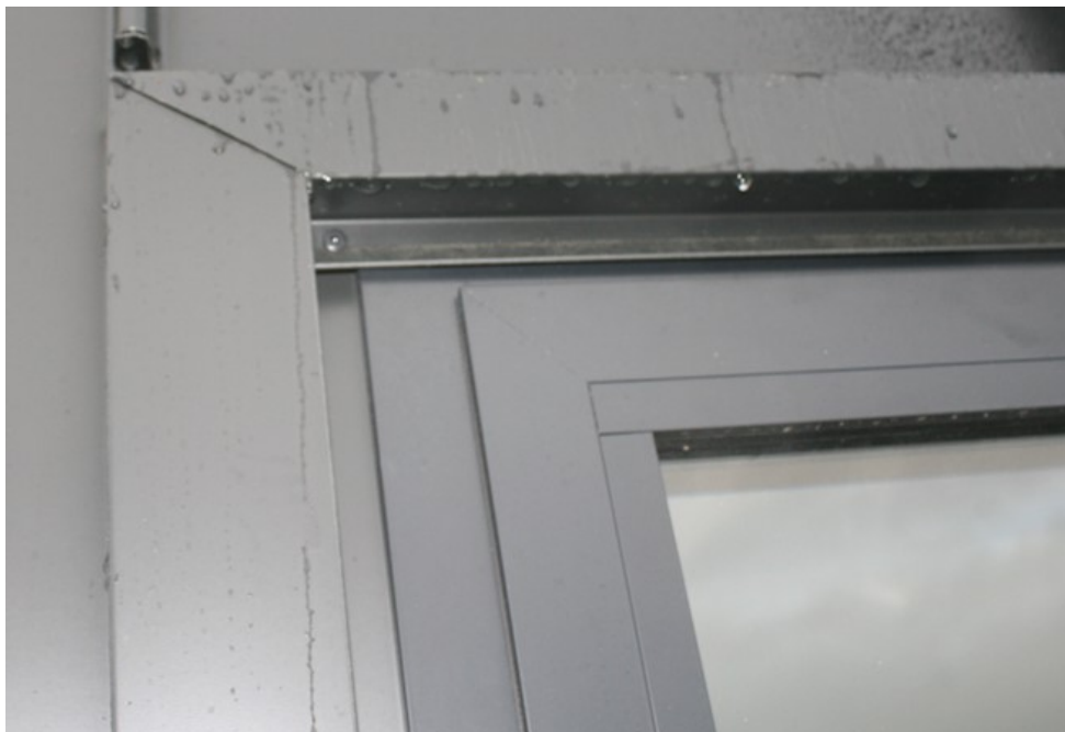
Using clipped flashings to minimise the use of rivets is a feature of a well-installed standing seam roof.
